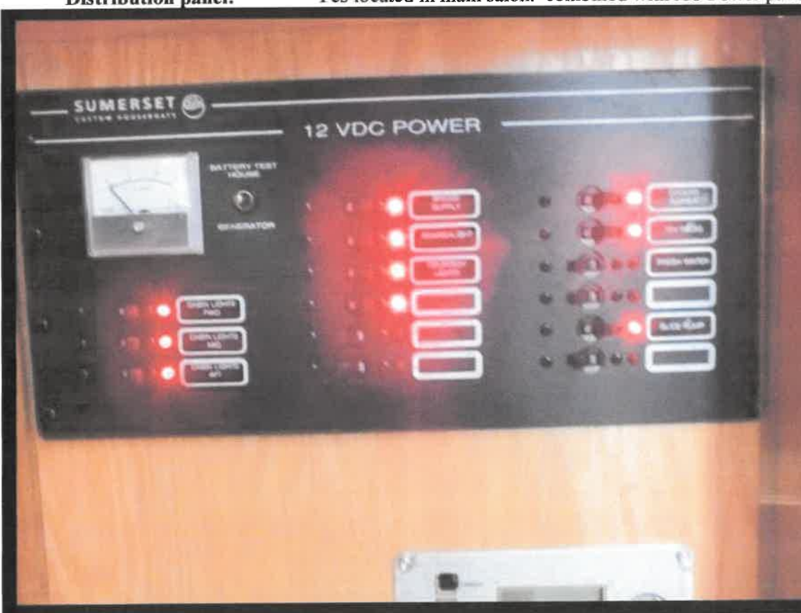
Breaker(s)/fuse(s): All D.C. circuits are adequately protected by branch breakers.
