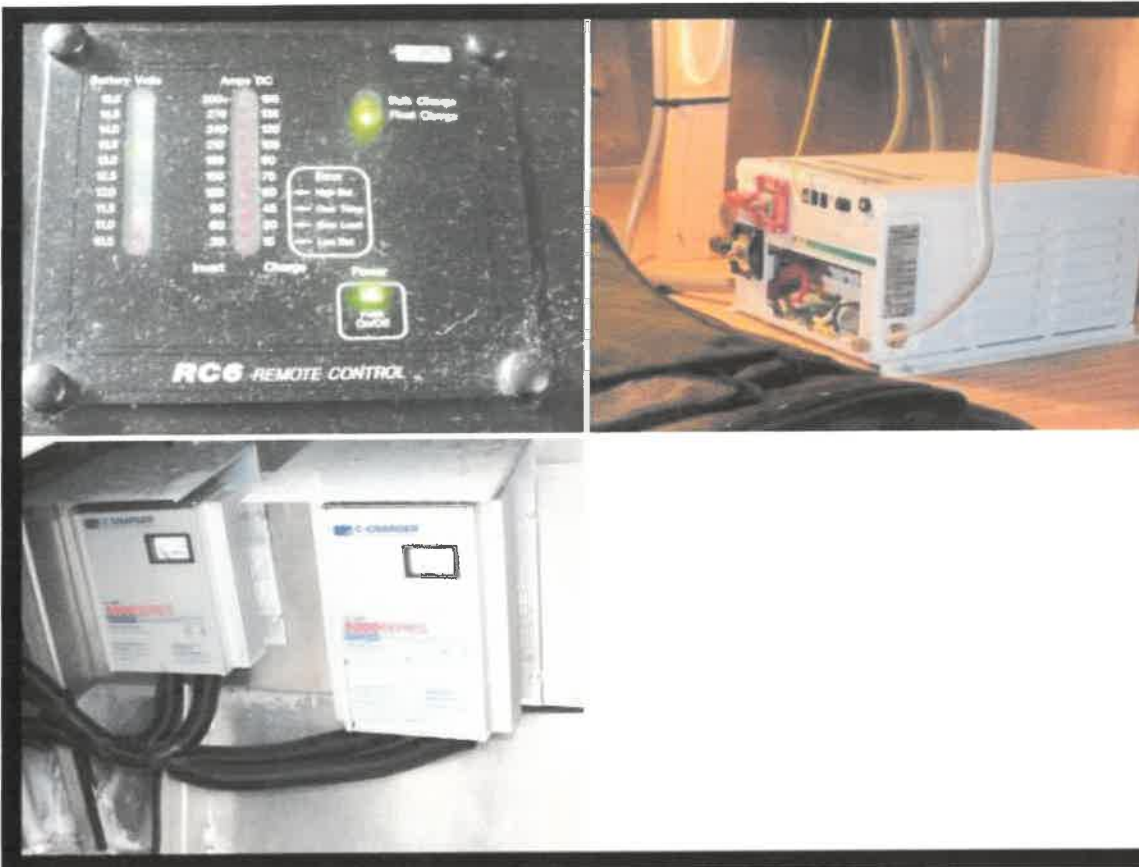
Distribution panel: Yes located in main salon. combined with AC Power panel.
