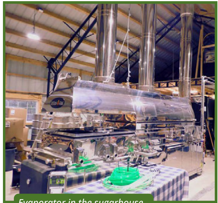
Evaporator in the sugarhouse.
